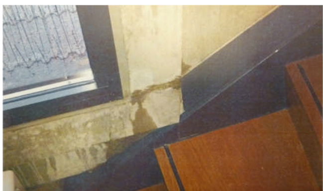
Foto 2.15: Lekkages 23-10-2010 – betonnen kaders.
